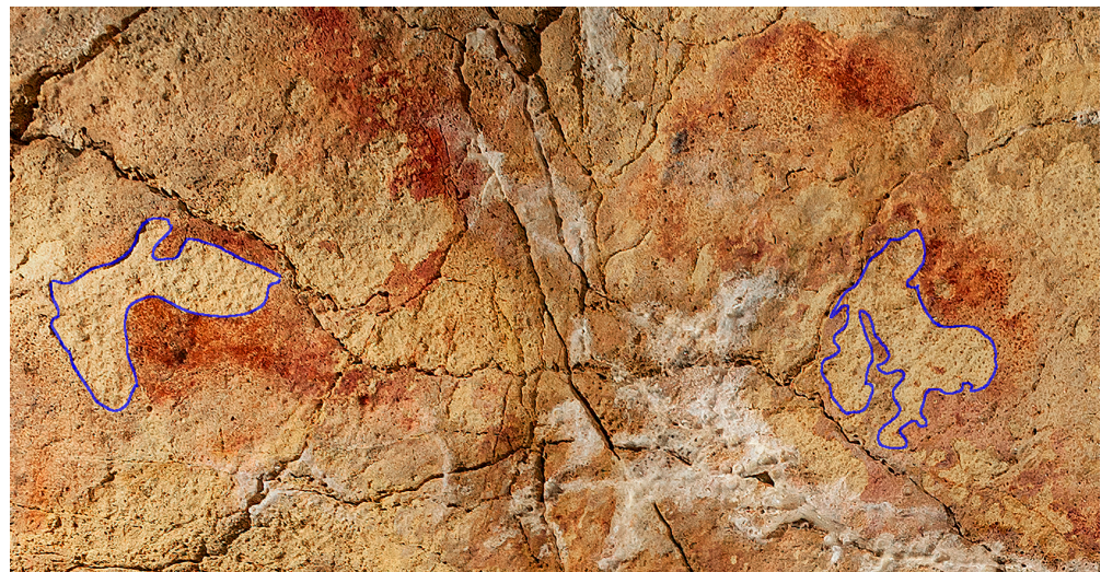
Figure 8. Area of the ceiling of the Polychrome Hall affected by a marked lack of support. The areas highlighted in blue indicate a lack of supporting rock. Within these highlighted areas the washed pigment, washed away by the water, has been redeposited.
